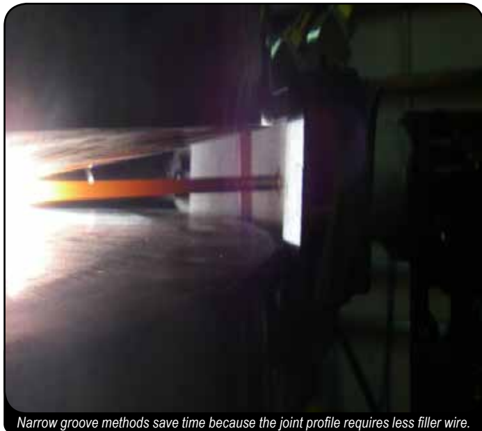
Narrow groove methods save time because the joint profile requires less filler wire.
